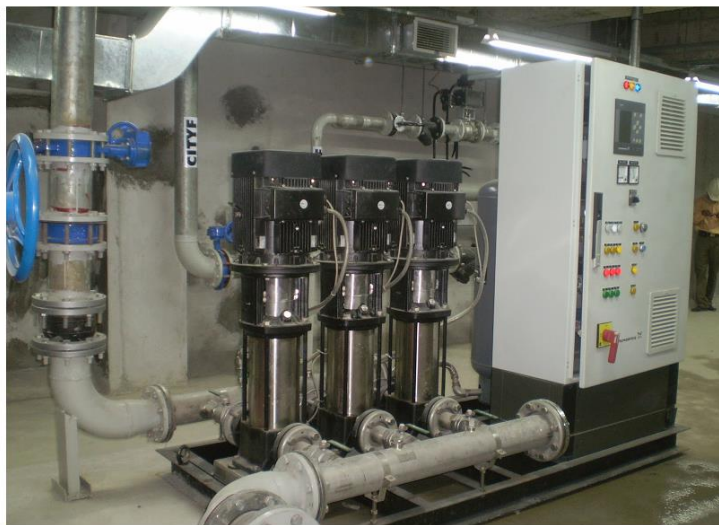
Water pump control panel
