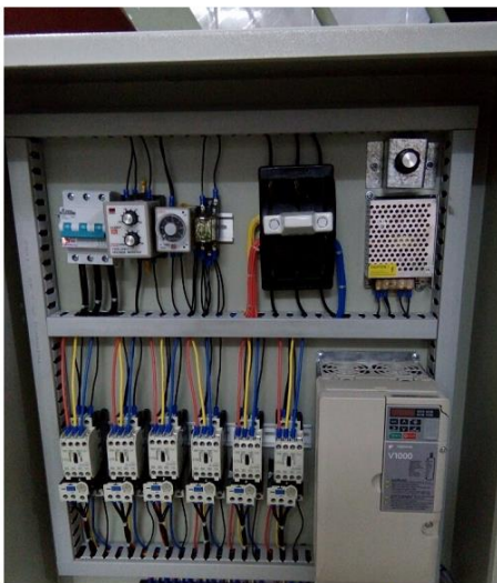
Inverter control panel
